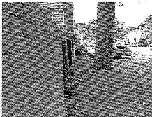
Garden wall pier leaning left, trunk leaning right (south).
