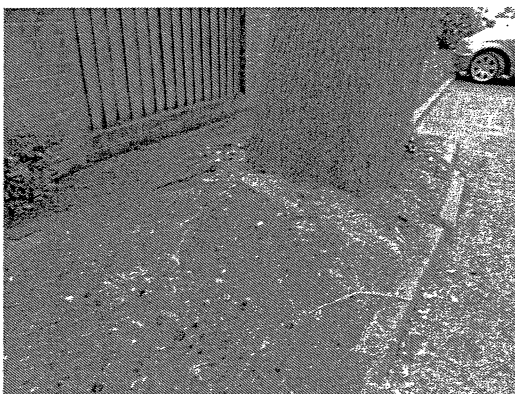
Base of trunk showing damage to pavement.
